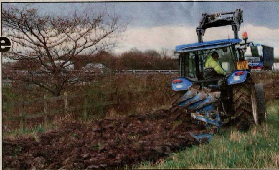
● ABOVE: Work starts to prepare the land off Hall Lane for the planting of thousands of trees to create Griffin Wood.
