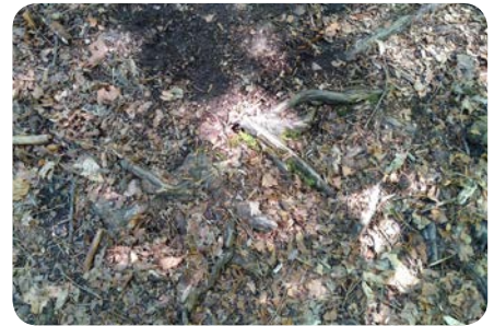
Photograph 3: Floor overgrown with roots
